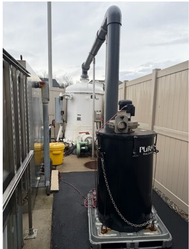
Scrubber Unit and Ecoverde Start Up at Lift Station 17
