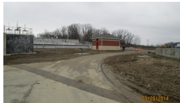
Final grading underway at the treatment plant, looking southwest at the VLR control building and new VLRs.
