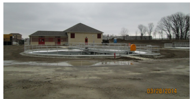
Looking east at the new Clarifier 6 and the blower room addition in the background.
